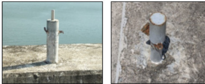
Figure 6. The crest Settlement staple cover is not installed and the padlock is broken
