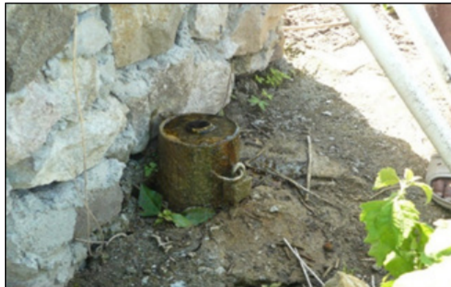
Figure 3. Water overflows in SP.4
